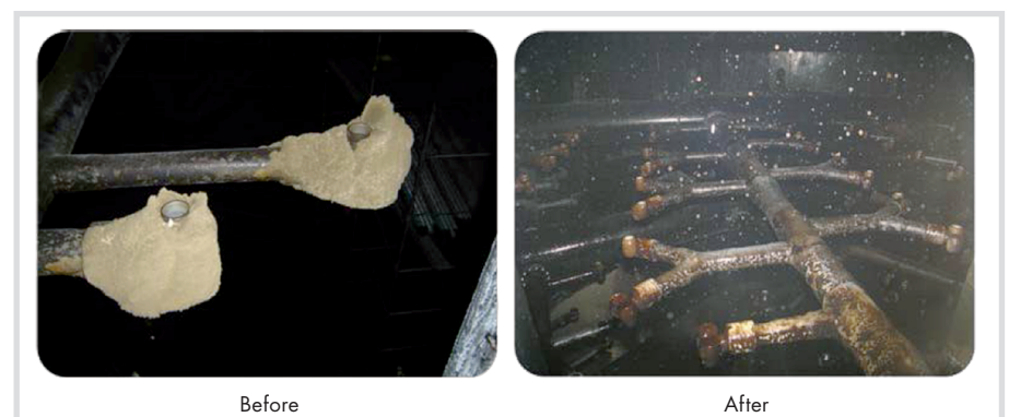
Fig. 2 Deposits around the nozzles were eliminated after modification of the spray system.
